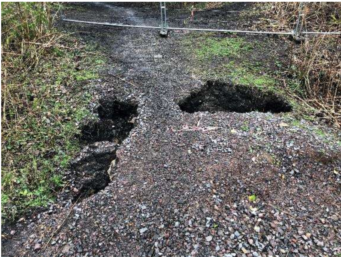
Plate 2: Collapsed section of footpath above dilapidated culvert conveying Nant y Groes.
