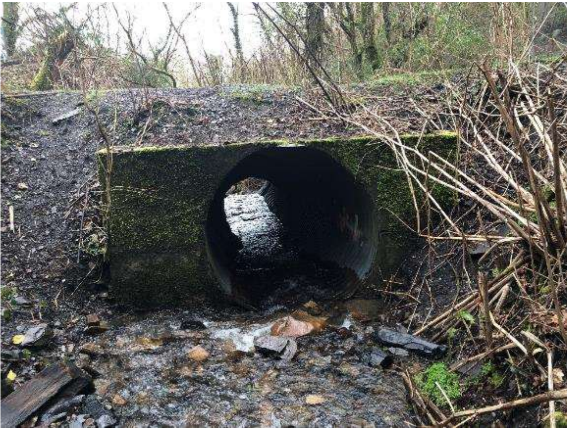
Plate 3: Head wall of Nant y Groes culvert on eastern side of the tip.
