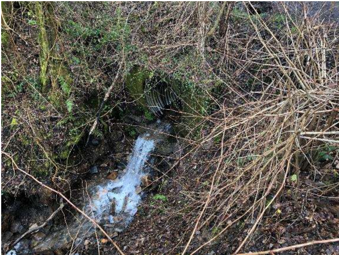
Plate 1: Nant y Groes conveyed by culvert on the eastern side of the tip – localised scour.
